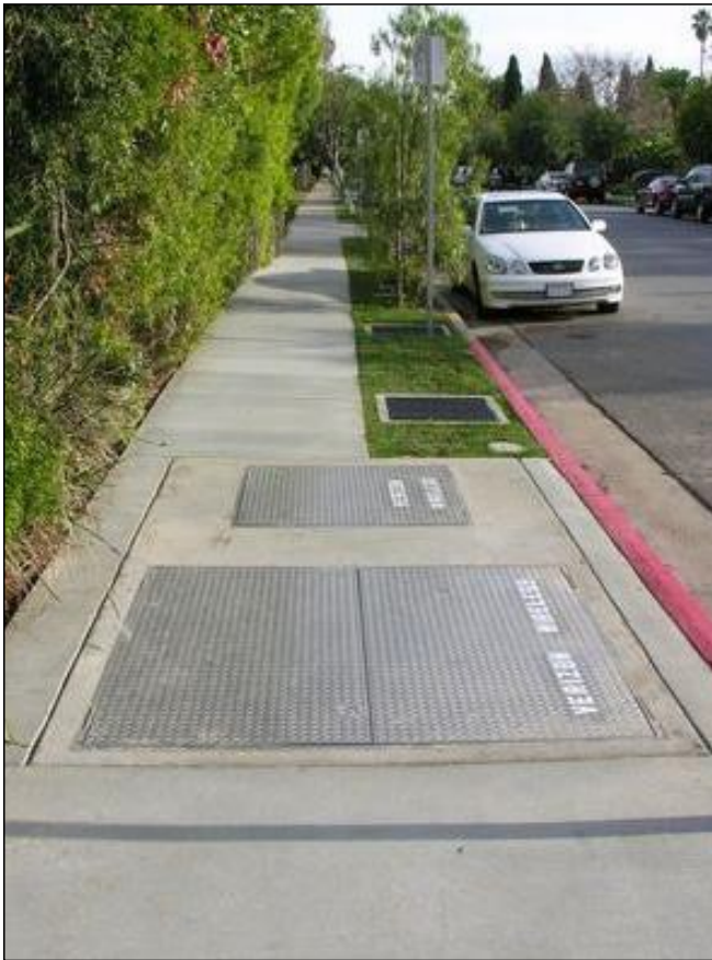
Figure 3: Flush-to-grade underground equipment vault.
