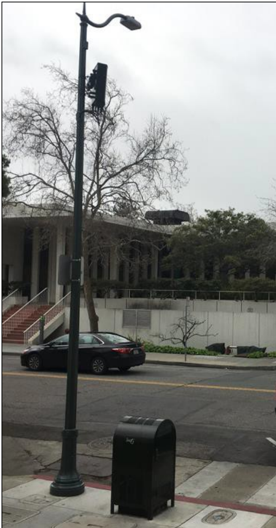
Figure 7: Ground-mounted accessory equipment concealed as a mailbox.
